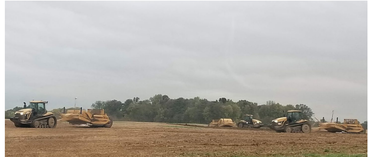
Yellowbud Solar Project
