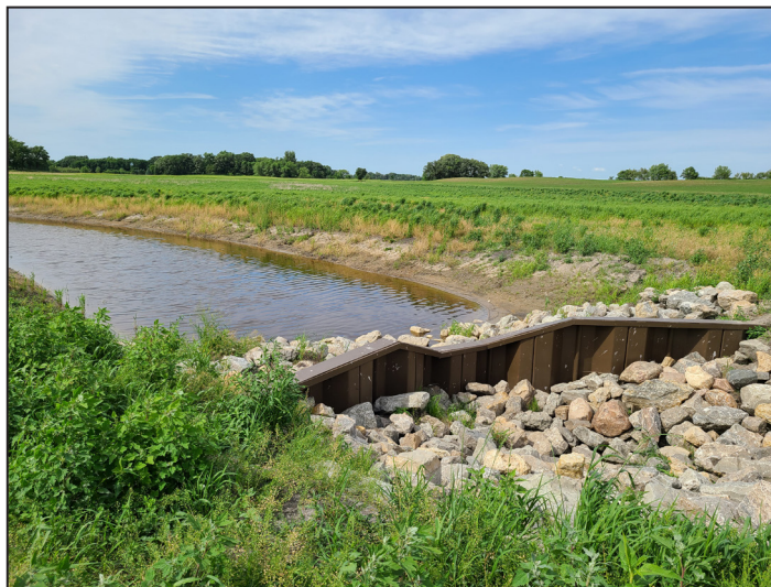
Above: An outlet structure installed on a Freeborn County MN CREP easement provides water storage. Photo Credit: Freeborn SWCD
