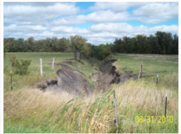
Erosion site identified and prioritized by the Erosion Site Inventory in 2010.
