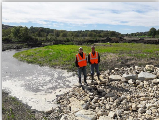
Skip Langer of the Olmsted County Soil & Water Conservation District, left, and Glen Roberson, Technical Service Area 7 Administrator Goodhue County Soil & Water Conservation District, made a site visit during construction of a project that will reroute a stream prone to erosion, and create a floodplain wetland habitat on the site of a former golf course in Rochester, Minnesota.
