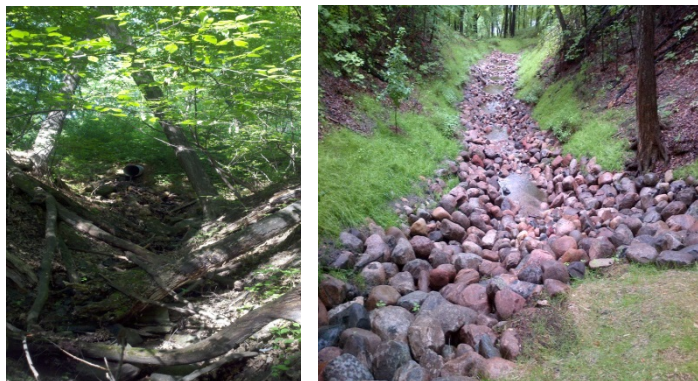
Left: Before project, eroding bank slopes. Right: After project, bank slope is stabilized.
