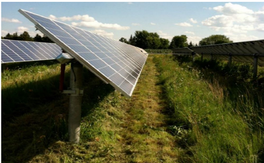
Mowing between solar panels.
