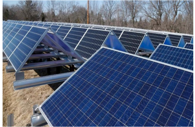
Dome-type solar panels – high areal coverage
