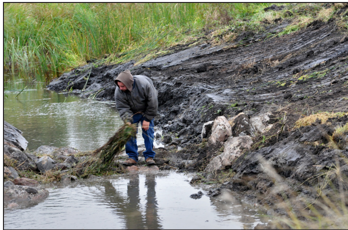
Top: Drywood Creek erosion control and habitat improvements will keep an estimated 212 tons of sediment — 16 dump truck loads' worth — out of the river annually. Bottom: A corn field obscured contractors' work.
