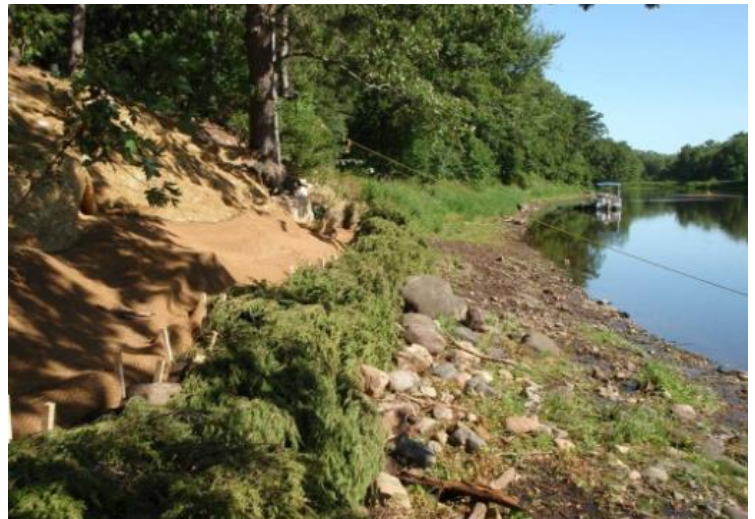
Bank stabilization with cedar revetments and erosion fabric along the St.Croix River
