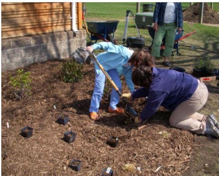
Raingarden where mulch has been applied before planting to prevent compaction Photo: Metro Blooms
