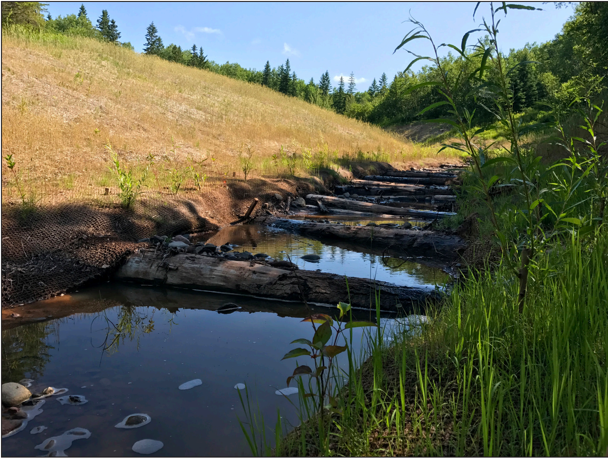
Aspen logs stacked two high and anchored by rocks form steps in a 500-foot-long segment of remeandered stream. Technical Services Area No. 3 staff engineered the project.
