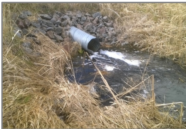
Figure 1. Upstream Drainage Tile Outletting into Restored Wetland
