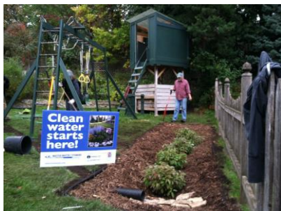
Stewards Dave Stack (R) and Jacquie DiGiacomo finish up installing a rain garden in a neighbor's yard.
