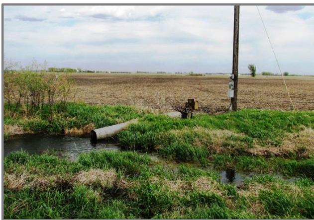
Figure 3. Low Lying Tile Drained Wetland Landscape Aided by Electrically Powered Lift Station
