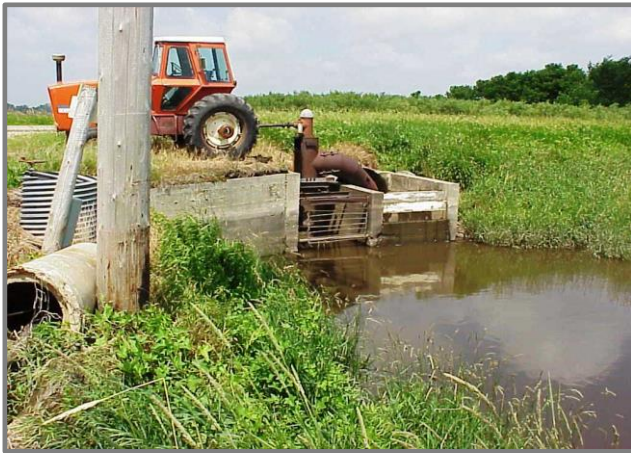
Figure 2. Drainage Pump Powered by Tractor's PTO
